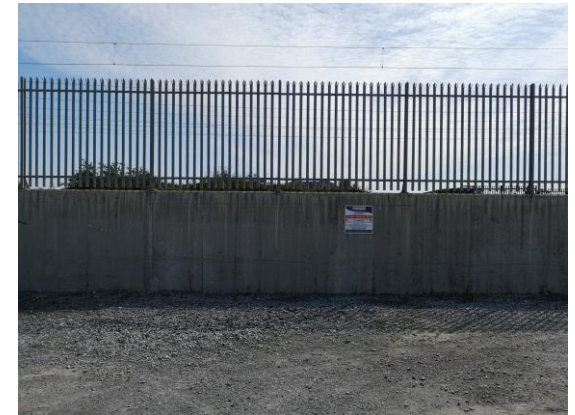
2. Existing Front view of Rail boundary. 2m Reinforced Concrete wall with 2m security fence (approx.).
